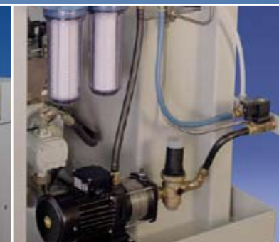
Optimum feed water supply with booster pump and double filter.
